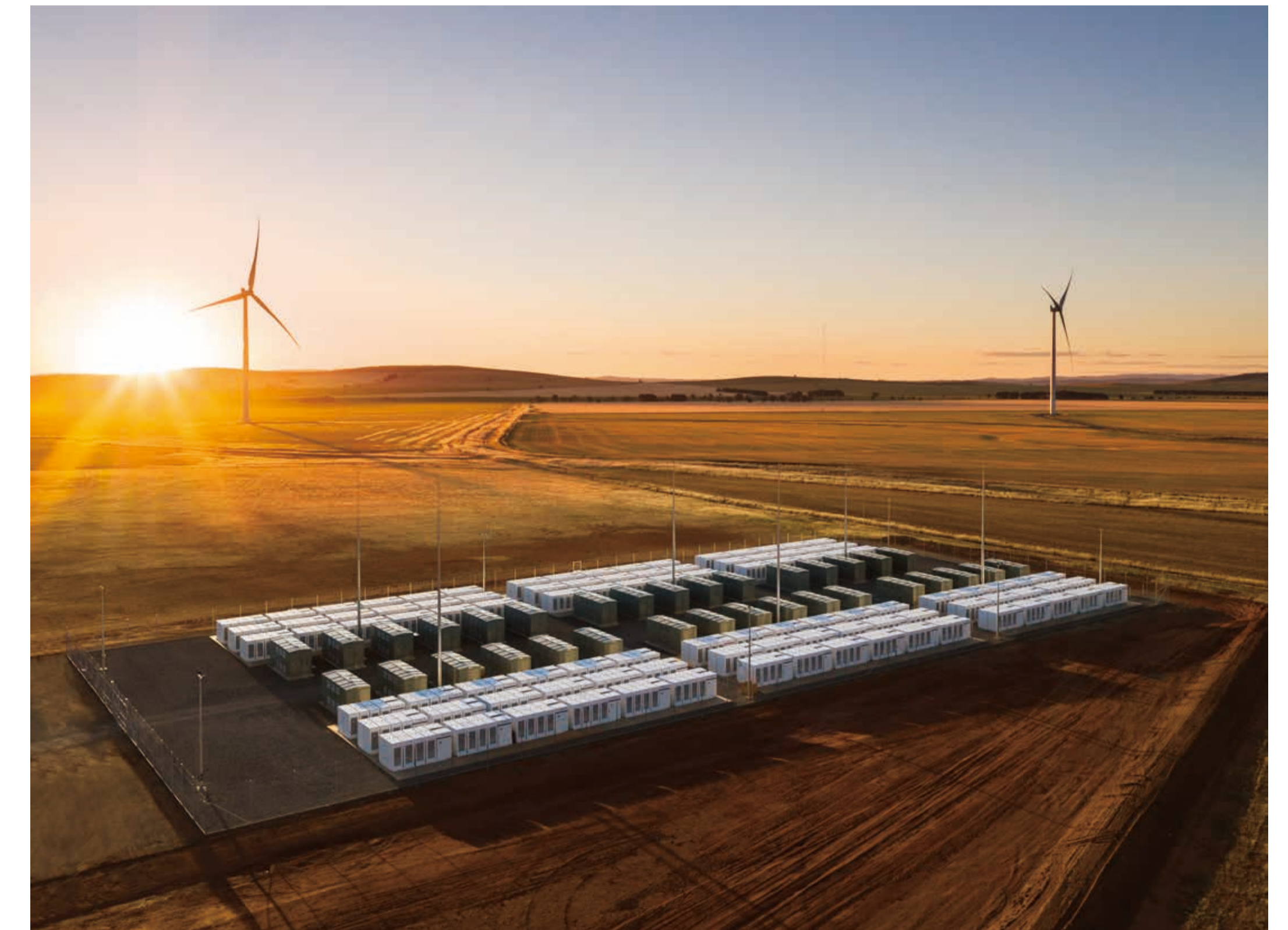
View of the battery system and wind turbines
